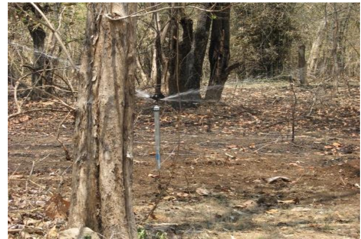
Sprinkler for raising fodder plot – A new addition to the existing system
