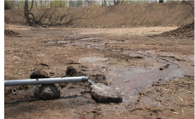
Water outlet from over-head tank flowing into the percolation tank
